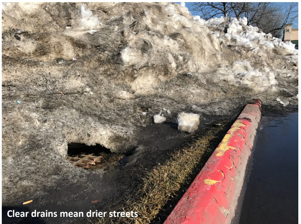
Above: Storm drain partially blocked by ice and snow
