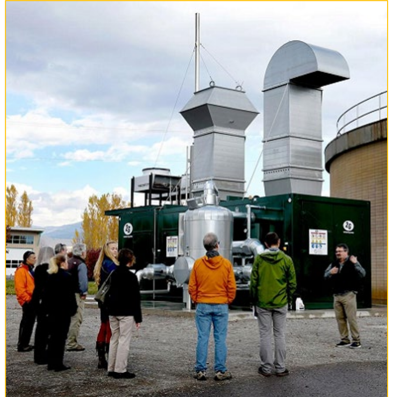
The bio-generator at the Resource Recovery Facility creates electricity from the methane produced from the sewage treatment process.
